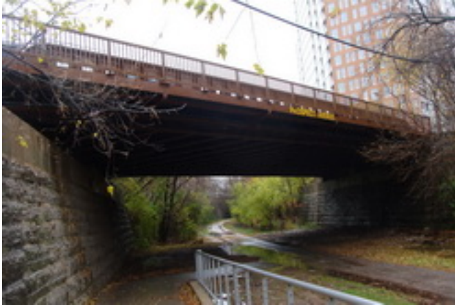
North Prospect Avenue Bridge over Oak Leaf Bike Trail, Milwaukee County, WI
